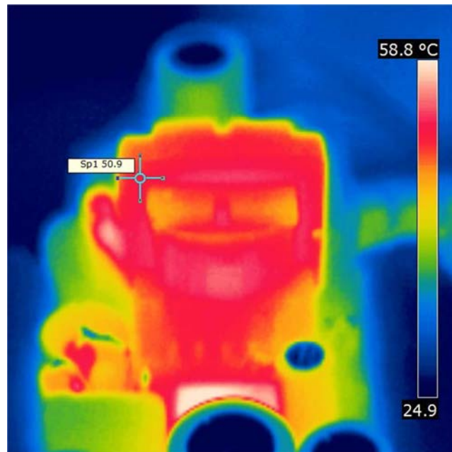
Figure 25 – SP1 – Transformer (T1).
